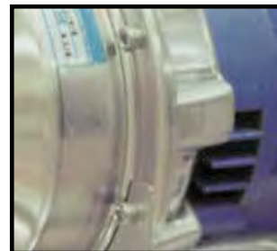
Typical pump casing bolt
